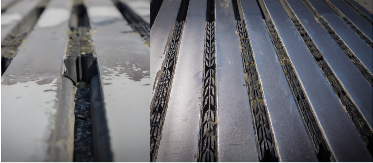
Figure 4-11. Over one month of installation, gravel and debris started to fill up the unsupported portion of the joint (left), while we observed no debris in the chevrons themselves. While the chevrons remained in good condition, some foam had been pulled from the supports after one month of wear (right).
