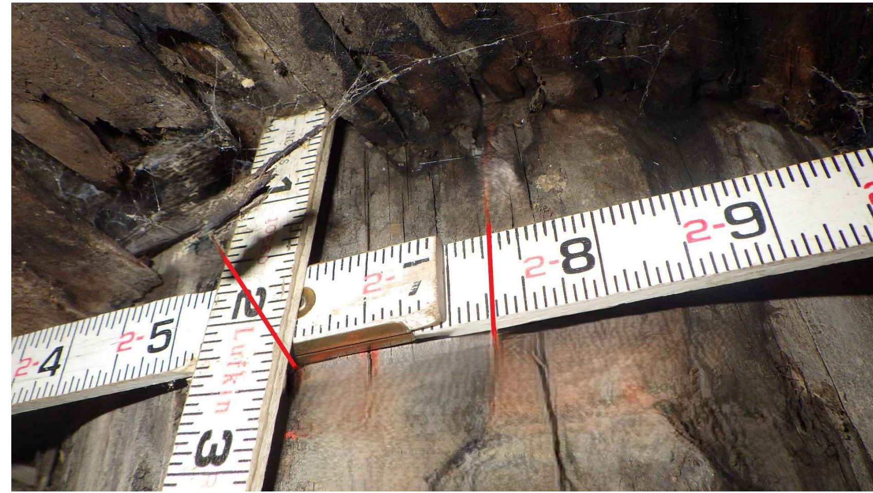
2 PHOTO - DAMAGED AREA S-1 NTS
