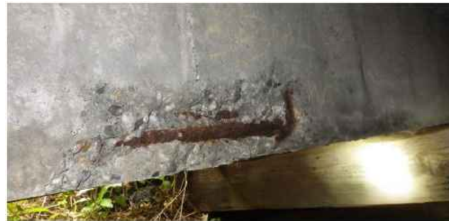
7 PHOTO - SPALLED CONCRETE AT TUB GIRDER S-1 NTS
