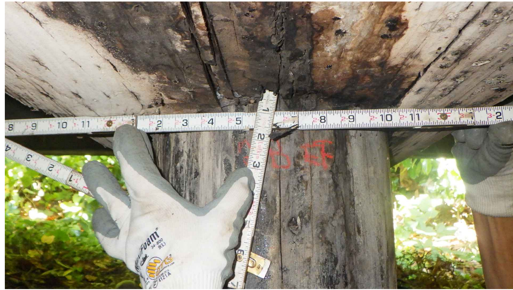
1 PHOTO - DAMAGED AREA S-1 NTS
